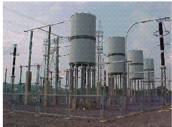
Fig. 7 - ELETRONORTE 550kV CLR at site
