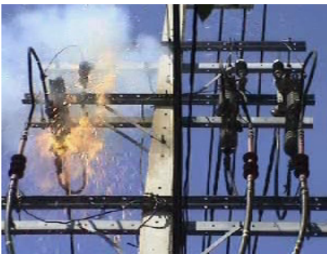
Fig. 7. A photograph during arrester failure of phase R
