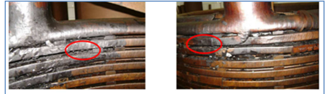
Fig. 3. Internal part of the high voltage winding indicating the failure
