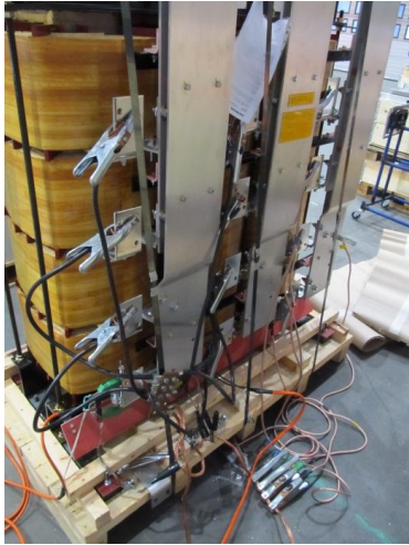
Fig. 9. 4.5 MVar reactor with measurement equipment attached.
