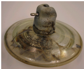
Fig. 11. Damaged insulator at 38.16 miles from the Goshen terminal.
