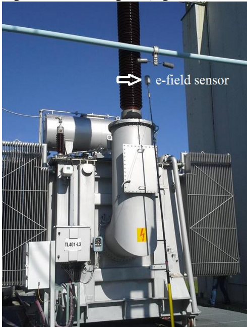
Fig. 3 E-field sensor at the 420 kV reactor
