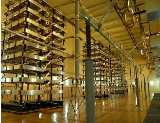
Fig. 1: IFA2000 valve hall after refurbishment.
