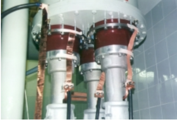
Fig. 5. Detail from testing: interconnected GIS enclosure and cable terminals
