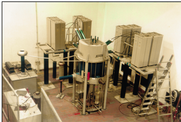
Fig. 2 Impulse current generator, TU-Graz
