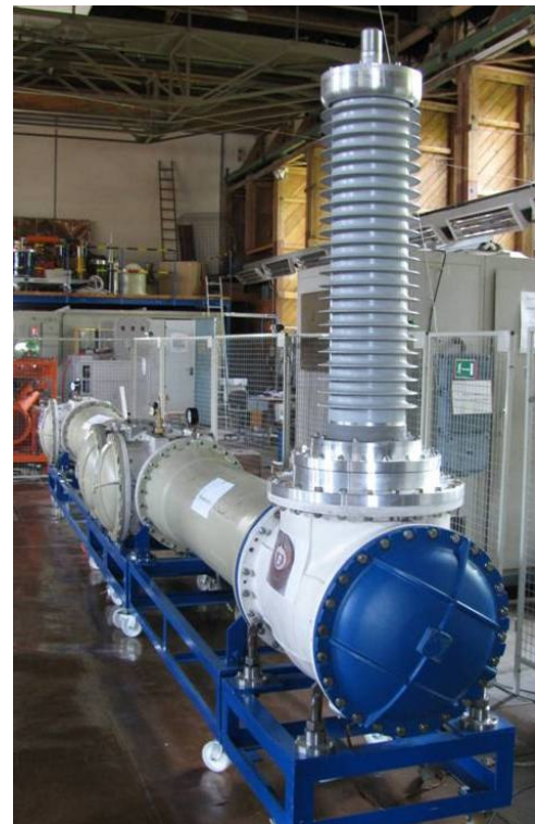
Fig. 7. The ABB 550kV GIS type ELK-3 for testing purposes at the University of Stuttgart.
