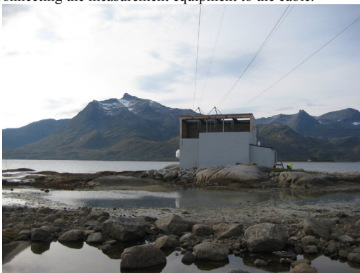
Fig. 8. Cable termination house.
