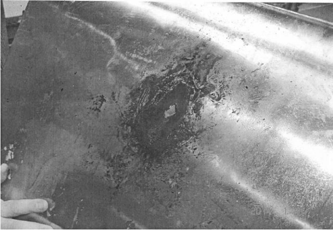
Fig. 2. Burning of the first layer of the LV foil winding
