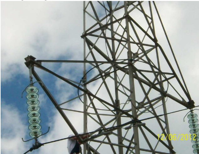
Fig. 1. Monitoring of the towers with the Rogowski coil.
