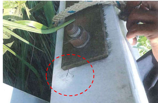
Fig. 9. Surface tracking at middle crossarm
