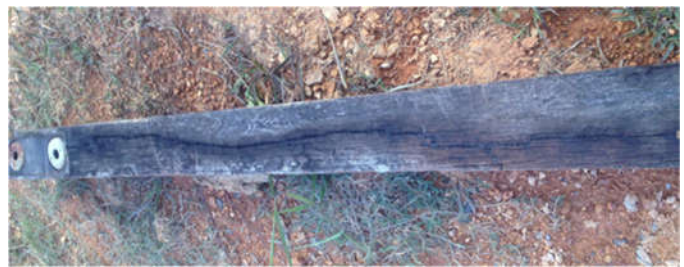
Fig. 1. Failed wooden crossarm due to lightning strike (Picture courtesy of TNB Asset Maintenance from 132 kV Kuala Krai to Gua Musang line outage due to lightning)
