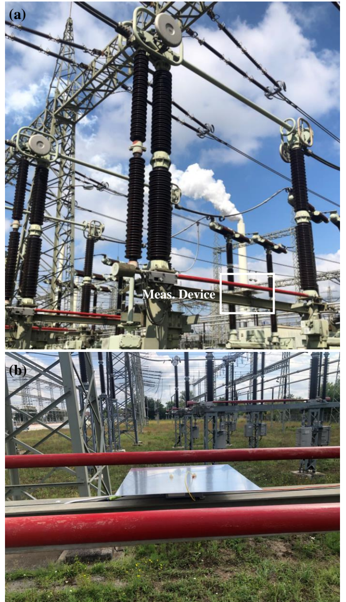
Fig. 8. Installation of the capacitive divider setups. (a) Overview of the installation. (b) Detail of one installed capacitive coupling plane.
