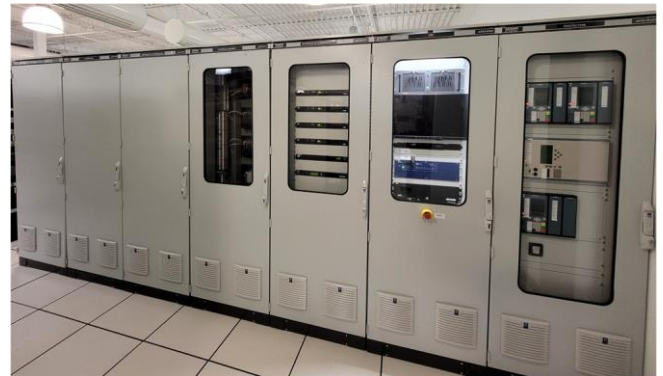
Fig. 3 La Verendrye control system replica in the HQ RT simulation laboratory (in IREQ).
