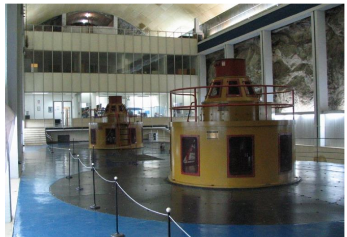
Fig. 1. The view of generators in the underground engine room
