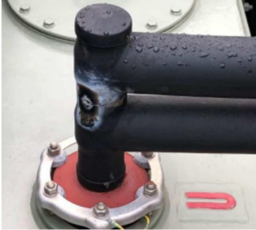
Fig. 2. Failed double cable connector at the 65 MVar shunt reactor terminal
