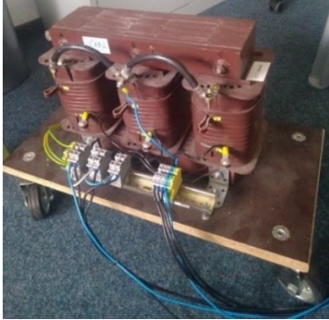
Fig. 5. Low voltage transformer with the vector group Yyn06
